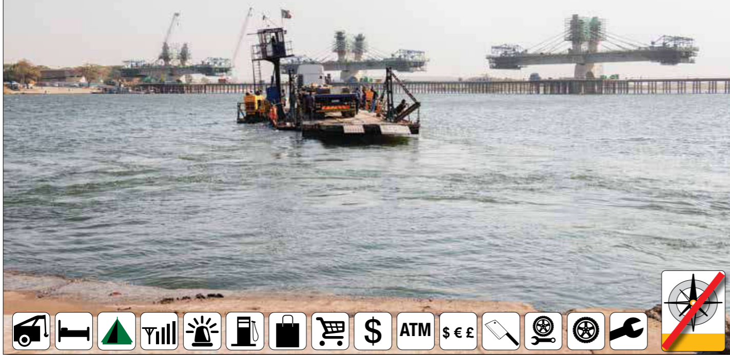
The Kazungula Ferry seen in the foreground will soon be replaced by the bridge you see being built in the background. (photo: Renzo Blasa)
