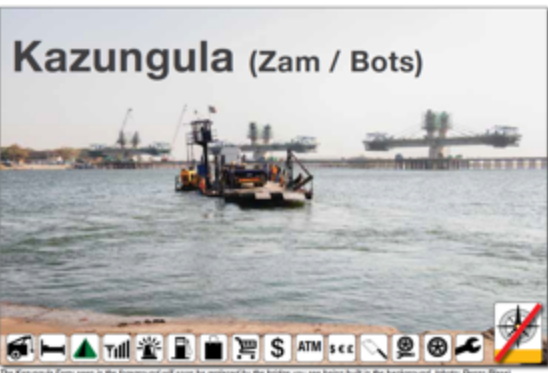
The Kazungula Ferry seen in the foreground will soon be replaced by the bridge you see being built in the background. (photo: Hans Dillinger)
